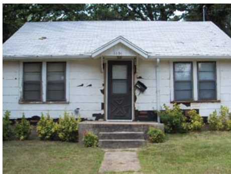
Moderate Housing Rehabilitation BEFORE
