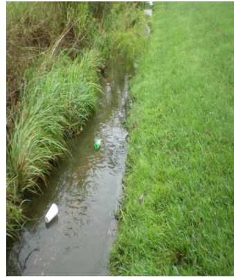
Trash in the concrete drainage ditch after going through the inlet.
