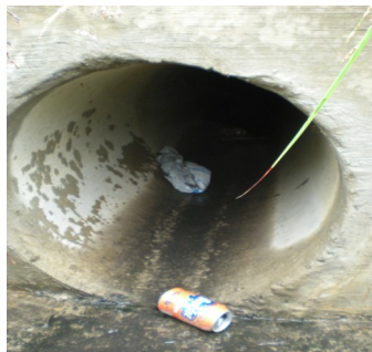
Trash at the outlet of a storm drain that leads to a creek.
