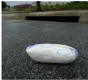
Dirty diaper in front of a storm drain inlet that leads to a creek.
