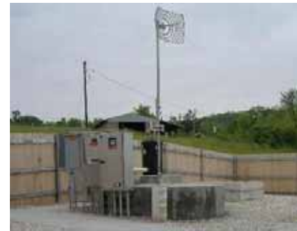
The Stonebridge Lift Station #13.
