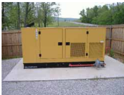
The generator at the Armstrong Lift Station #14.
